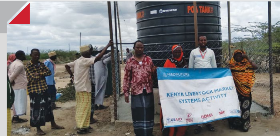
Members of Bura WPCs during the official opening of water tank installed at Garasweino Village (at the background) and the water standpipe for drawing water by community members.
