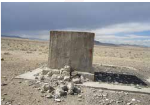
Picture 5. Khovd soum, Khovd aimag - the well before rehabilitation
