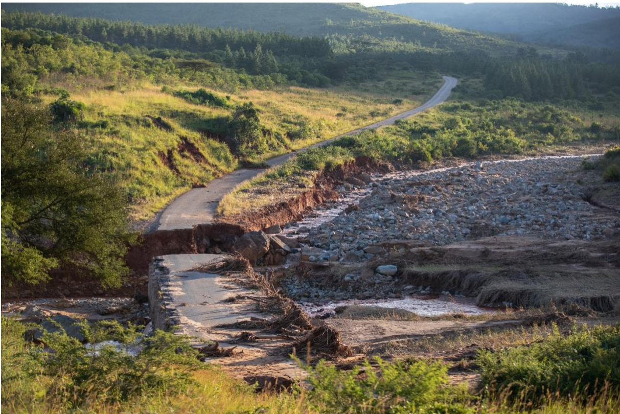
In Zimbabwe, washed out roads and bridges rendered some communities completely inaccessible after the storm. Ezra Millstein/Mercy Corps
